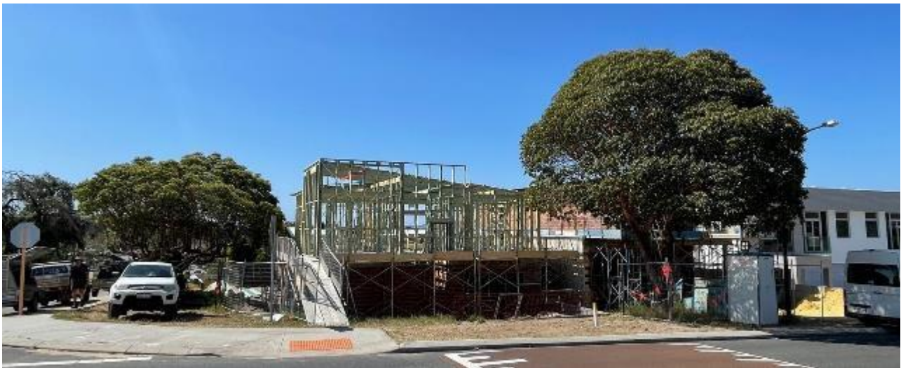
Figure 24. Residential development under construction with a larger footprint close to existing, mature street trees (Image Credit: Paul Barber).
