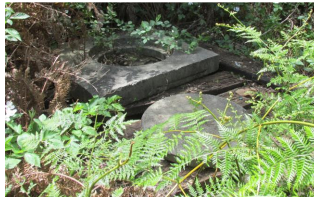
Old drainage cover overgrown with vegetation and in poor condition (Reg Bourke)
