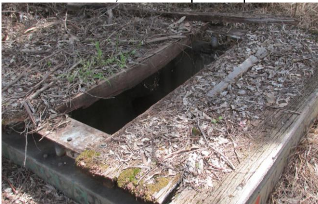
Broken cover over old drainage sump (safety hazard for fauna and personnel) (Reg Bourke)
