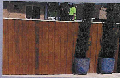
10D non-compliant ground levels
