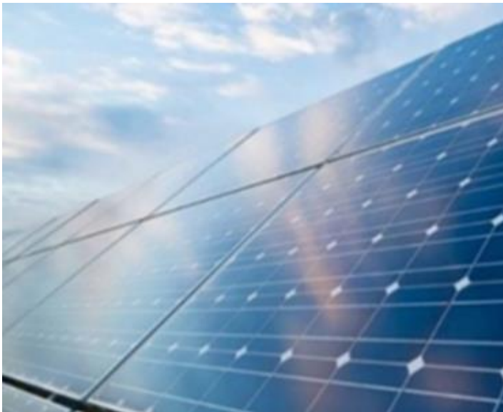
Figure 5-3 Rooftop PV system
