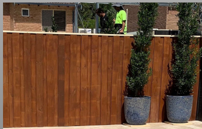
10D non-compliant ground levels
