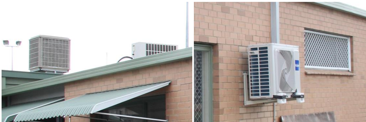
Figure 4: Photo 25 & 26 – Air conditioners
