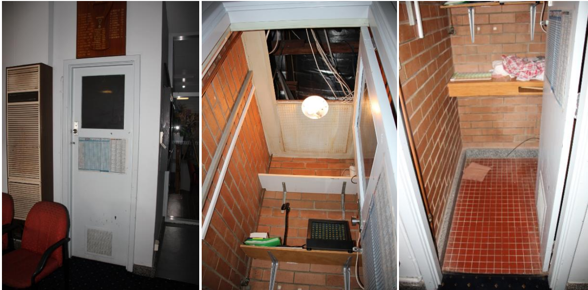
Figure 20: Photo 92, 93 & 94 – Electronics room
