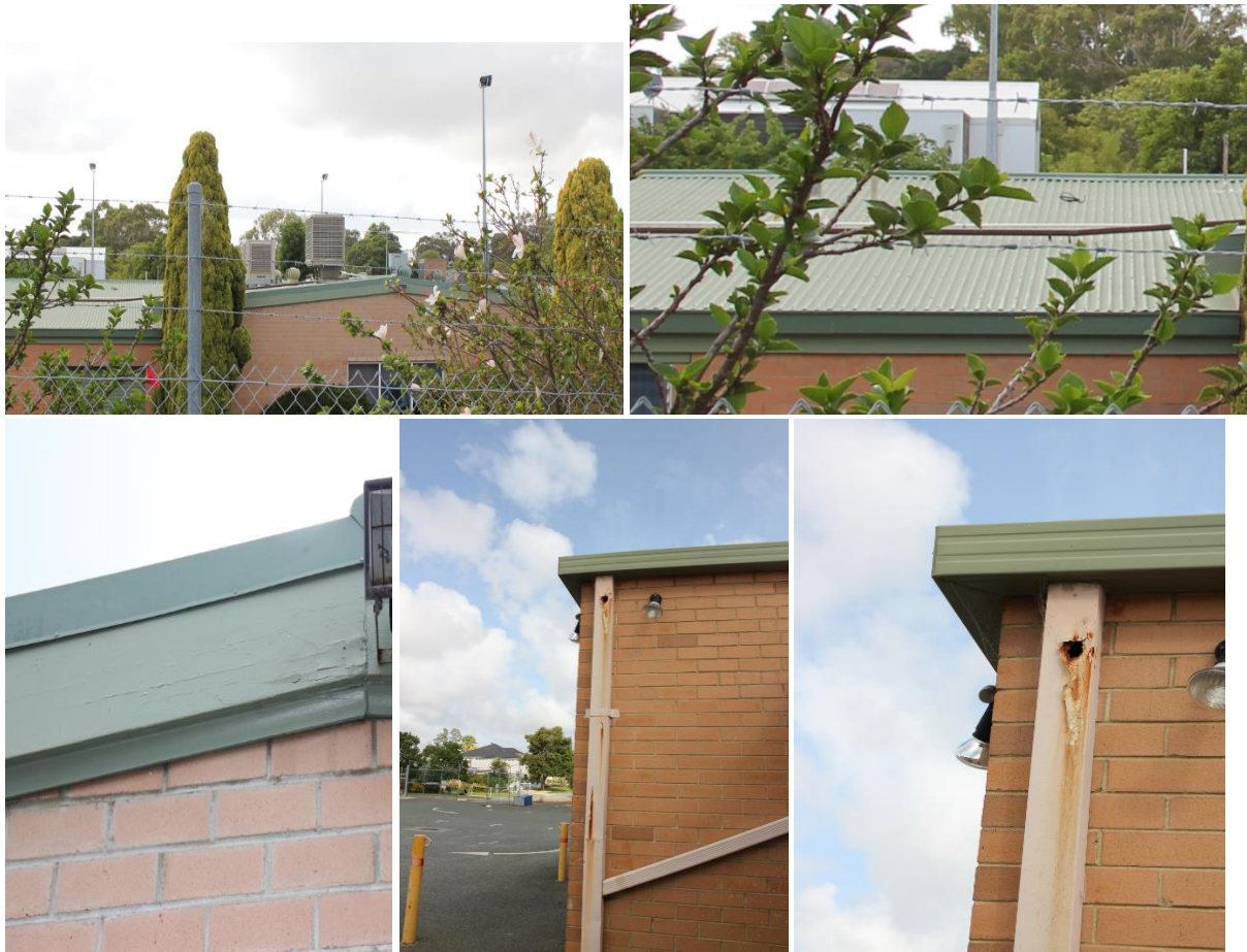
Figure 2: Photo 12, 13, 14, 15 & 16 – Roof cover
