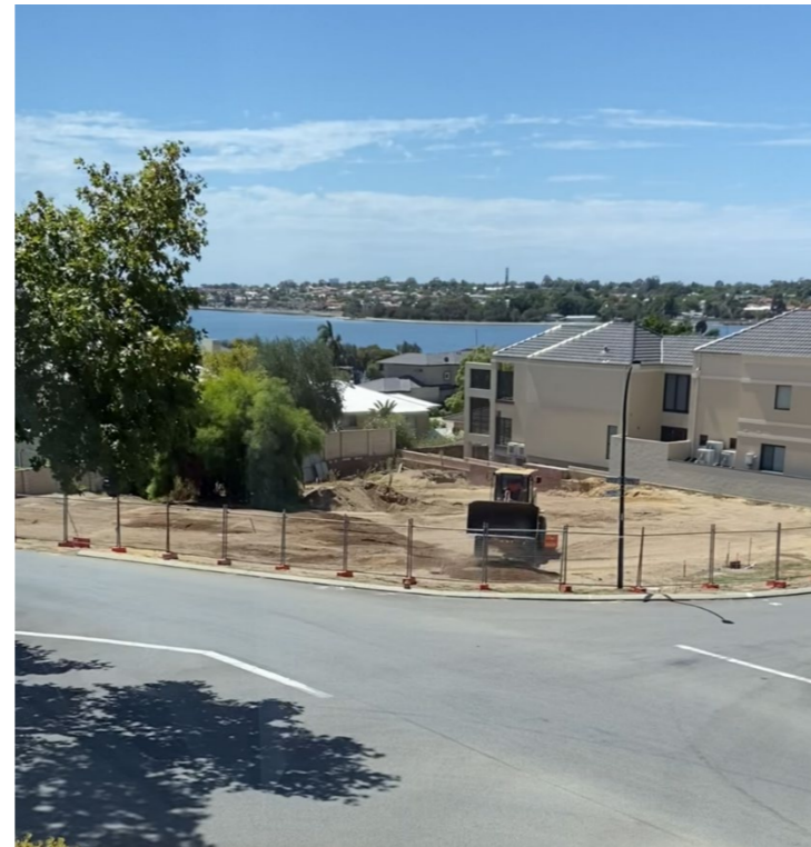
B) Video Still_Unauthorised Fill_13 March 2020 1rst sand mound levelled
