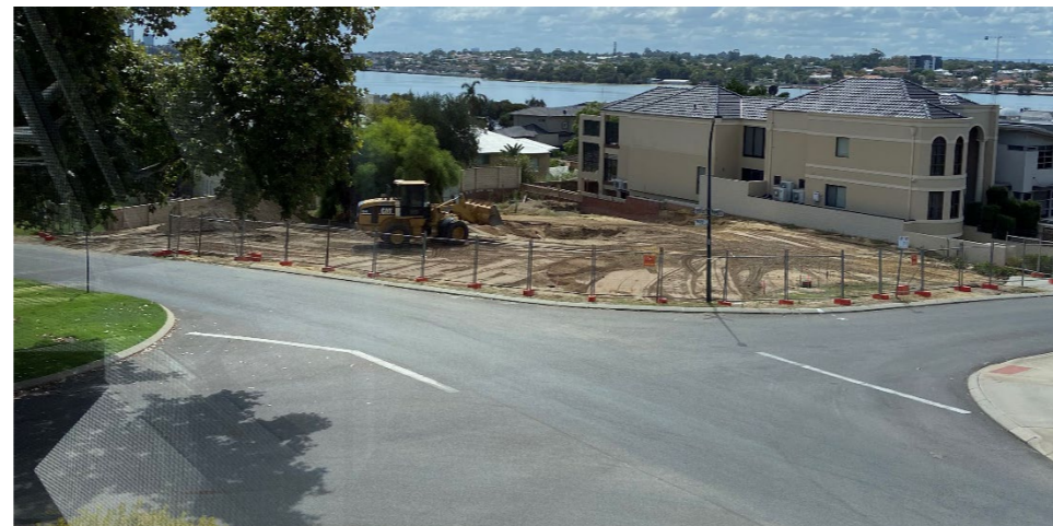
E) Photo_Unauthorised Fill_16 March 2020_10.50 AM 2nd sand mound added & levelled
