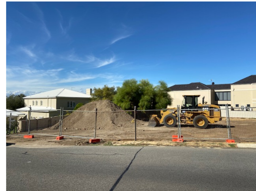
I) Photo_Unauthorised Fill_16 March 2020_3.15 PM 1 sand mound left standing
