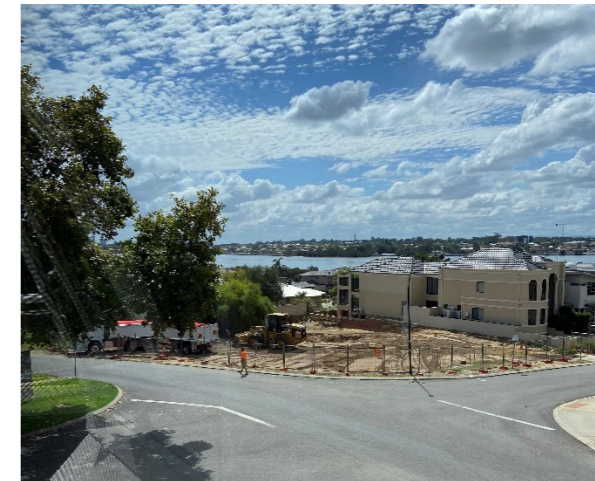
F) Photo_Unauthorised Fill_16 March 2020_10.55 AM 3rd sand mound added & levelled
