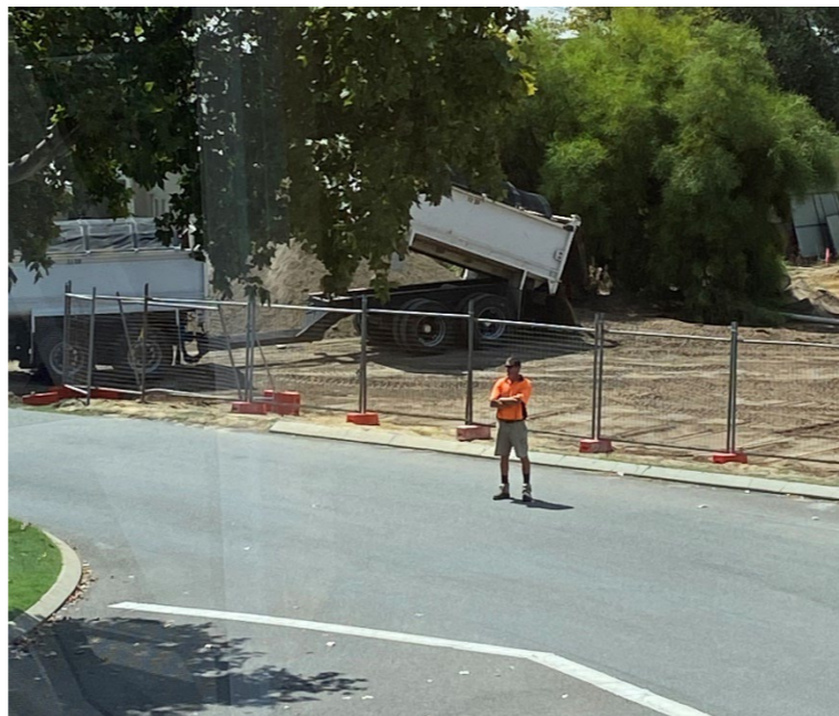
H) Photo_Unauthorised Fill_16 March 2020 2-3 more mounds of sand added & levelled
