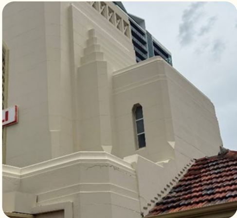
Figure 72 Cracking to the tower.
