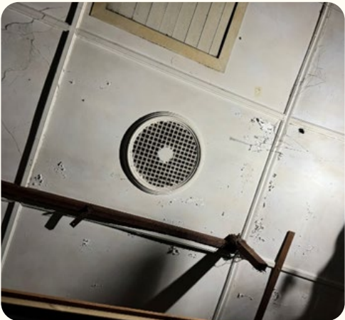
Figure 70 Paint peeling and cracks to the strapped ceiling above the stage.
