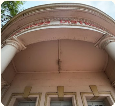
Figure 74 Substantial water staining to the entry portico.
