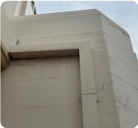
Figure 73 Cracking to the tower concentrated to areas near rainwater goods or the parapets which have ox gutters behind.
