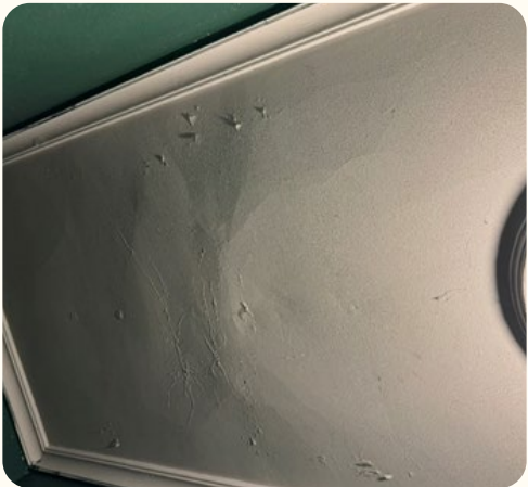
Figure 71 Water damaged ceiling in the north-west hallway.
