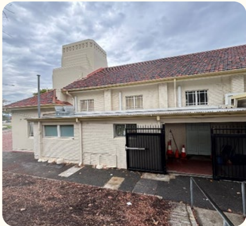
Figure 75 North-east elevation gutter to the auditorium roof has rusted out and slipped from the eaves.
