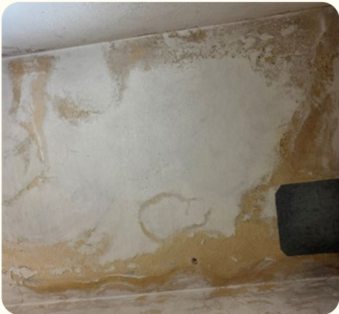
Figure 68 Historic water damaged ceiling to the tower staircase to the bio box.
