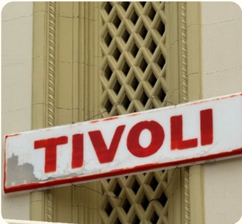
Figure 77 Tivoli signage is showing signs of wear
