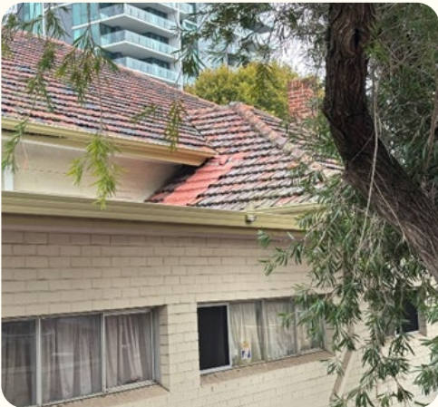
Figure 76 North-west elevation gutter has rusted out to the main auditorium and there are extensive flashings to the roof hip instead of downpipes or spreaders.
