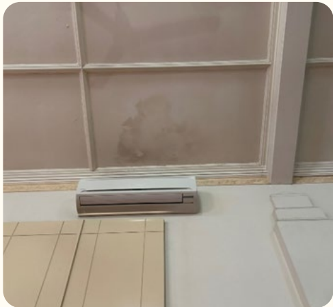
Figure 66 Water damage to the auditorium ceiling.
