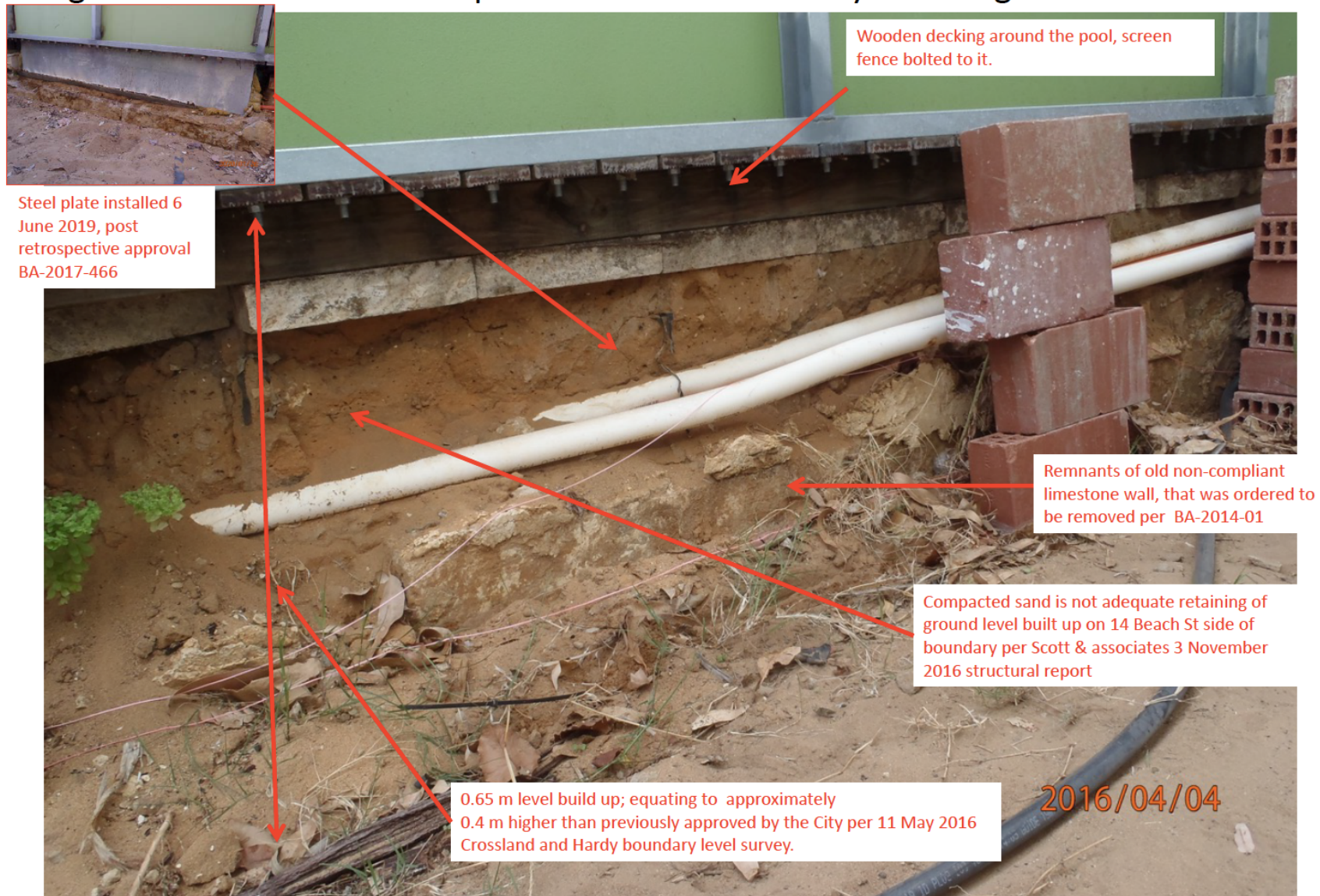
Figure 5.3 – 14 Beach inadequate limestone boundary retaining
