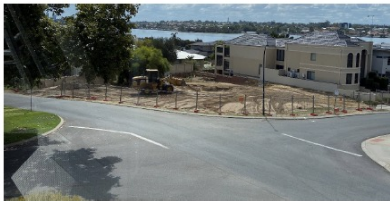
E) Photo_Unauthorised Fill_16 March 2020_10.50 AM 2nd sound mound added & levelled
