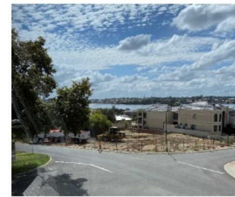
F) Photo_Unauthorised Fill_16 March 2020_10.55 3rd sound mound added & levelled
