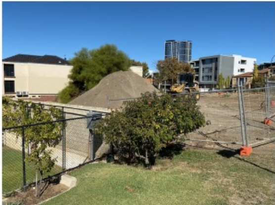
J) Photo_Unauthorised Fill_16 March 2020_3.15 PM
