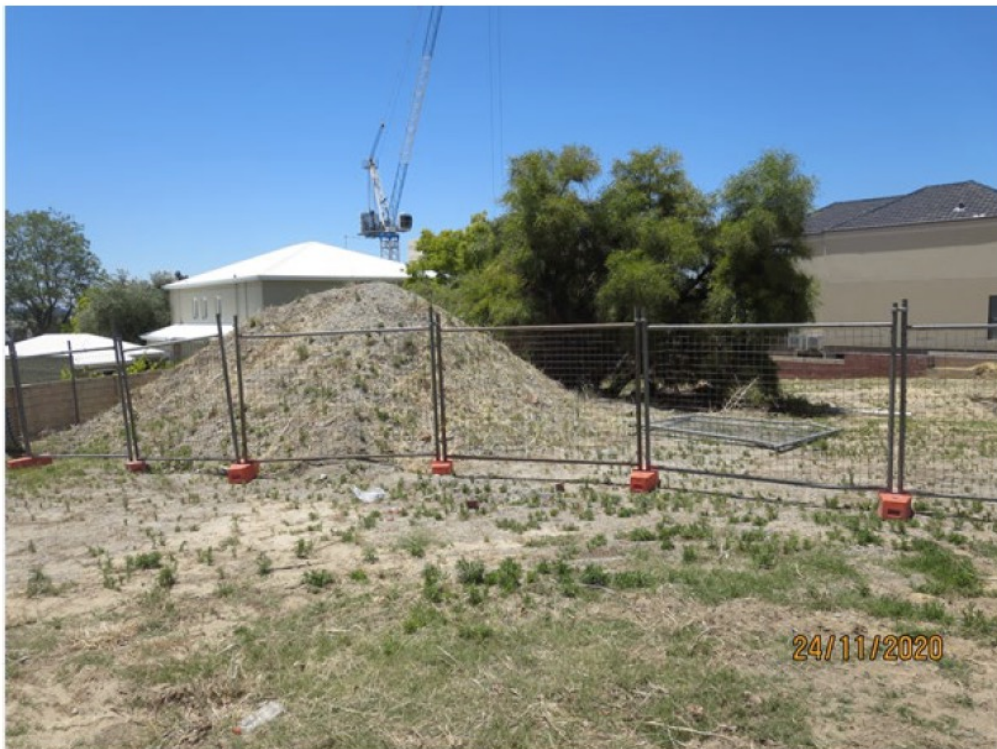
Photograph 1: Unauthorised material on site, November 2020
