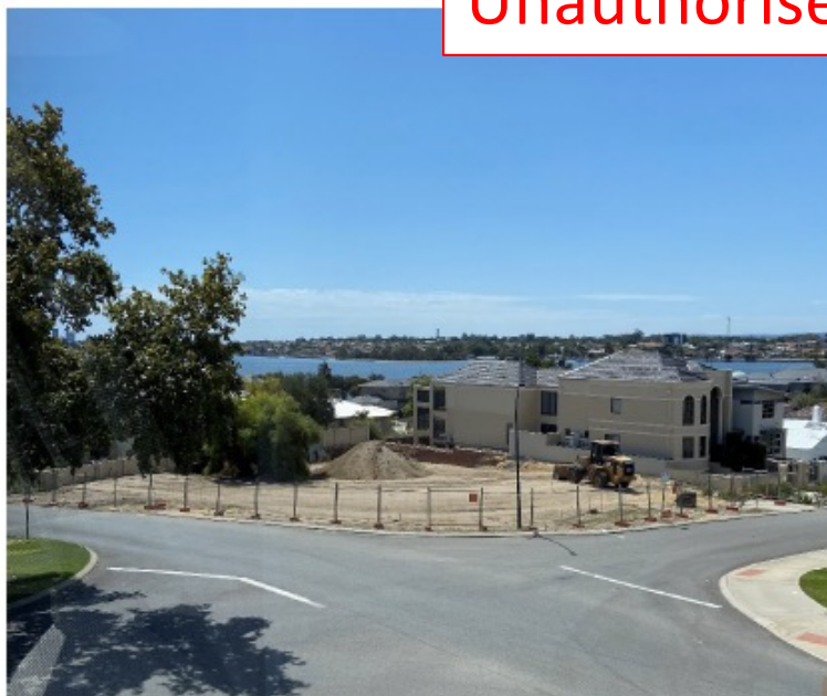
A) Photo_Unauthorised Fill_13 March 2020_11.45 AM_1rst sand mound added 1rst sound mound added
