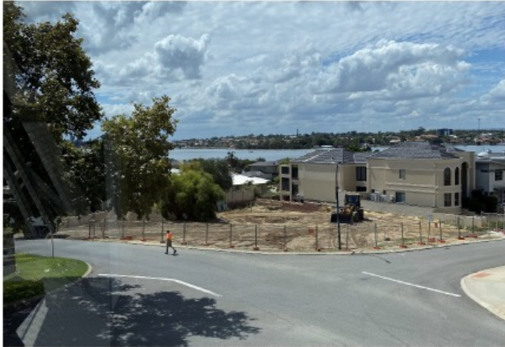
G) Photo_Unauthorised Fill_16 March 2020_12.30 PM
