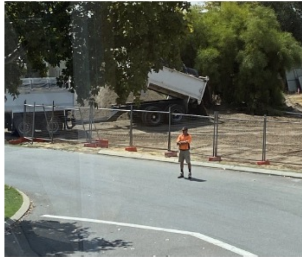
H) Photo_Unauthorised Fill_16 March 2020
