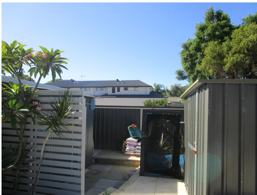
Figure 4: View of the neighbour's storage area which will abut the proposed kitchen boundary wall
