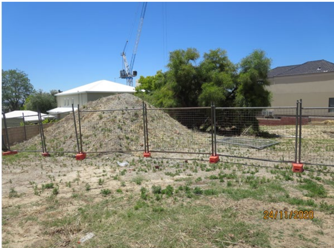
Photograph 1: Unauthorised material on site, November 2020
