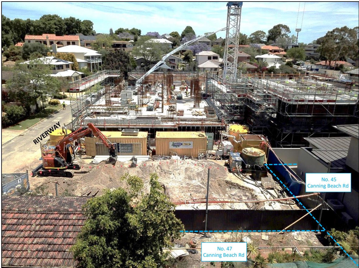
Figure 2 – HCACF Construction Site (View looking west from No. 47 Canning Beach Rd, Applecross, 19 November 2020)
