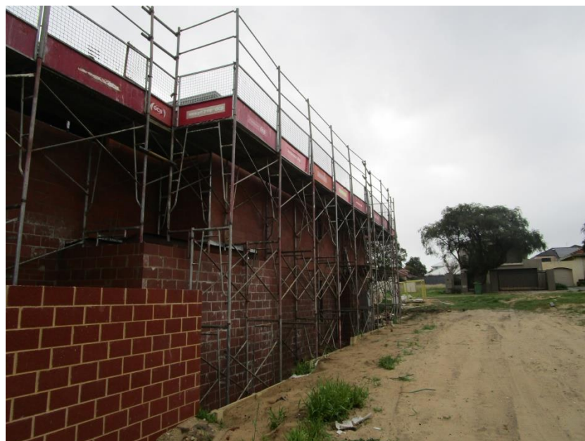
Figure 8: View northeast of the interface between the subject lot and the two storey house under construction at 36A Raymond Street.
