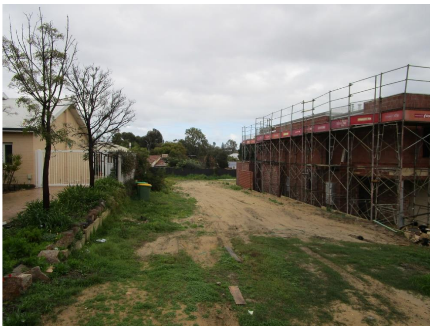
Figure 7: View of the vacant subject site. Note the difference in land levels between the subject site and the neighbouring properties on the left.
