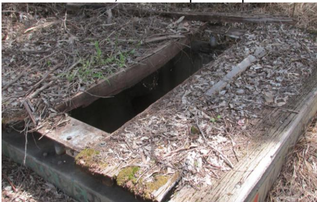
Broken cover over old drainage sump (safety hazard for fauna and personnel) (Reg Bourke)
