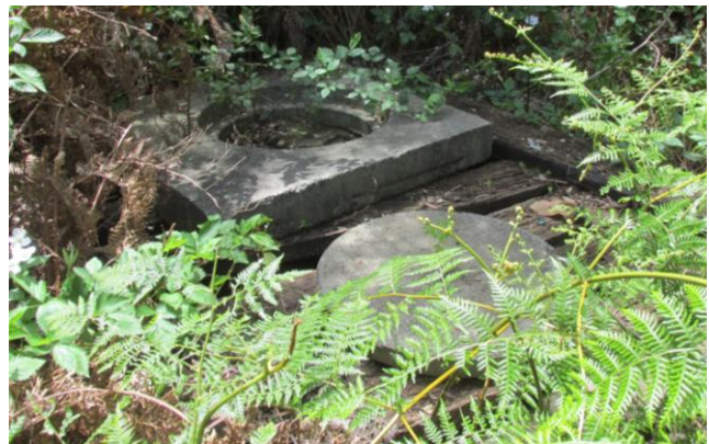
Old drainage cover overgrown with vegetation and in poor condition (Reg Bourke)
