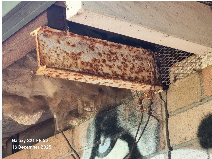
22. WESTERN ELEVATION - Eaves beam corrosion
