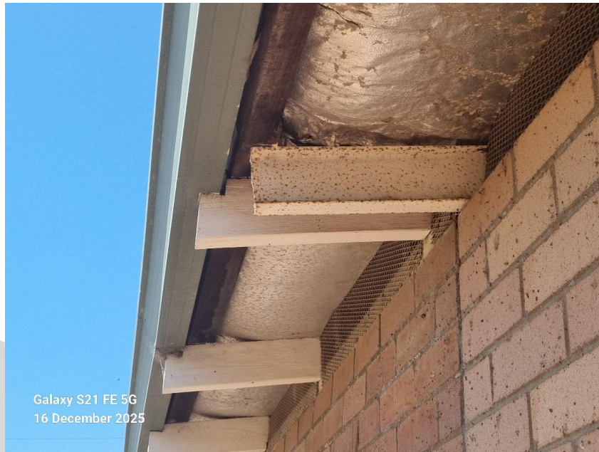
20. EAVES OVERHANG – Light corrosion on steel beam
