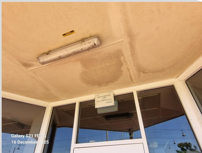
4. SOUTHERN ENTRY – Ceiling evidence of water ingress
