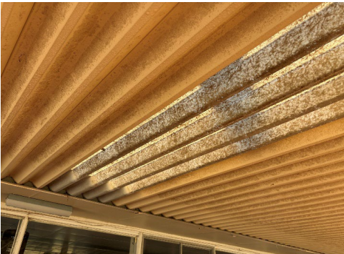
Defective opaque sheeting
