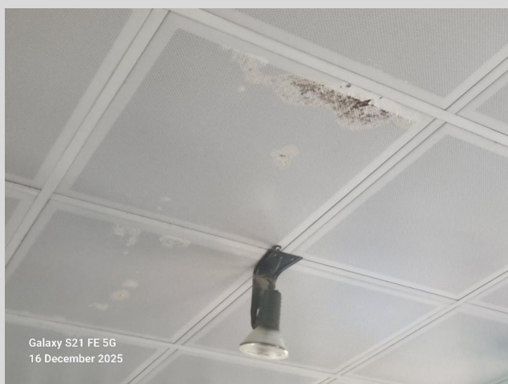
2. DANCE HALL – Evidence of Roof Leak
