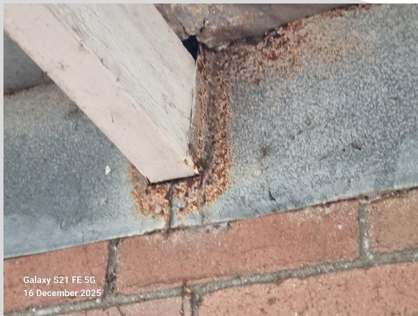
21. Corrosion of Flashing
