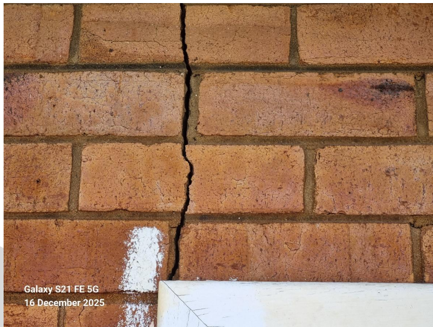
18. EASTERN FAÇADE – Large Brick Crack
