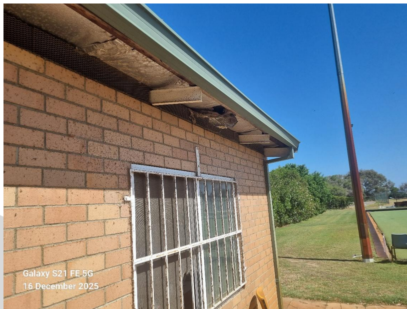
16. EAVES OVERHANG – Sarking torn under the eaves
