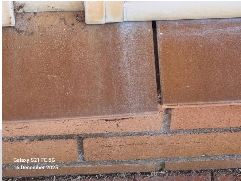
9. SOUTHERN ELEVATION – Loose sill tiles
