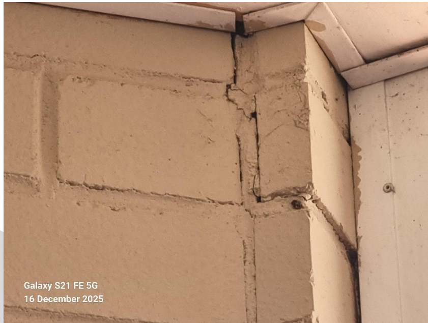
7. SOUTHERN ENTRY – Small brick crack
