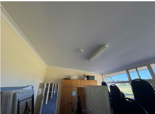
Storage room – defective ceiling
