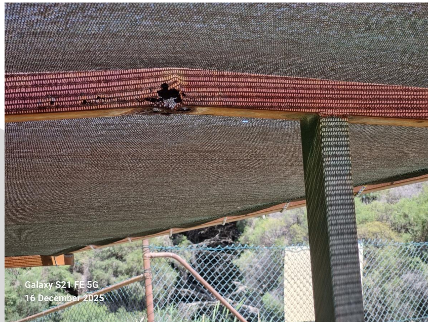
26. NORTH-WESTERN BOWLING GREEN – Failed member on shade structure
