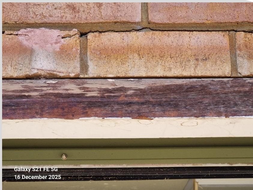
23. LINTEL – Minor brick cracking above door frame
