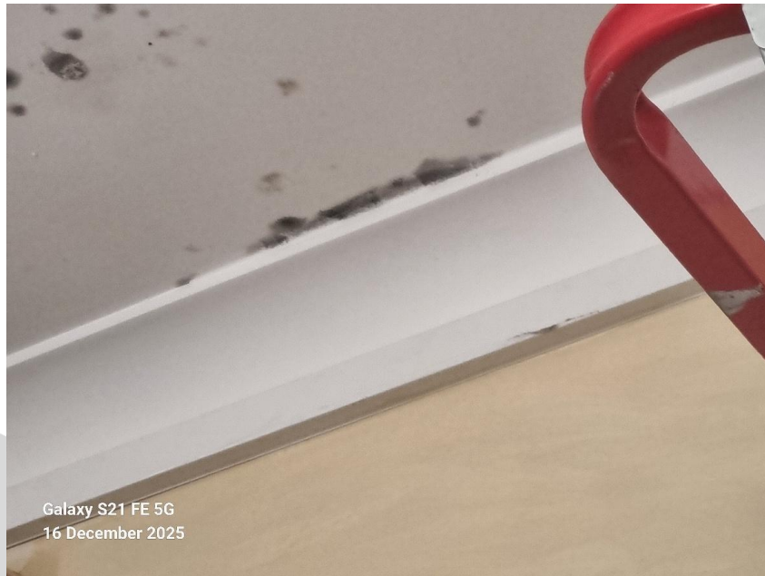
3. MENS LOCKER ROOM – Evidence of Roof Leak
