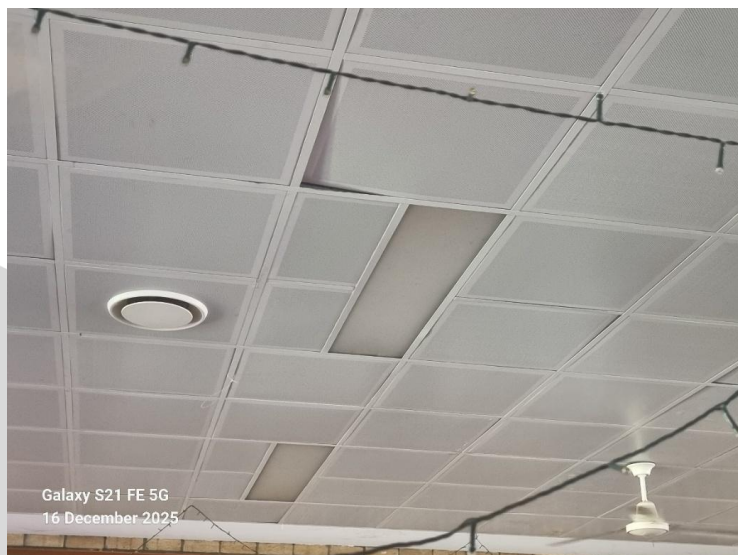
1. DANCE HALL – Loose Ceiling Tiles
