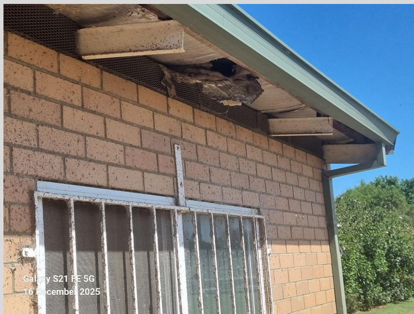
17. EAVES OVERHANG – Sarking torn under the eaves
