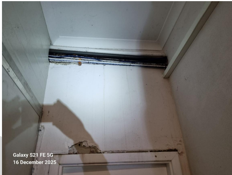
15. STORE ROOM – Condensate from pipes causing damage to door frame
