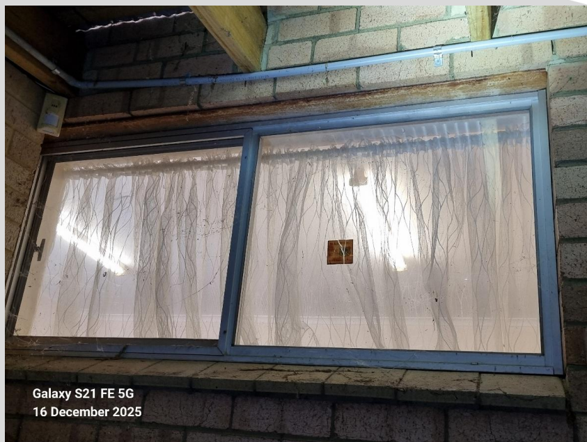
10. STORE ROOM – Corrosion of window lintel
