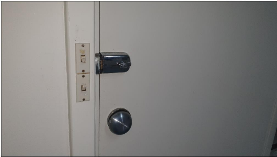
Ref # - 11 | Old style light switching to be tested
