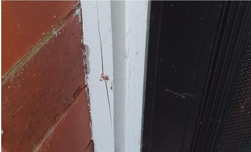
Ref # - 25 | Damaged Window and door frames throughout
