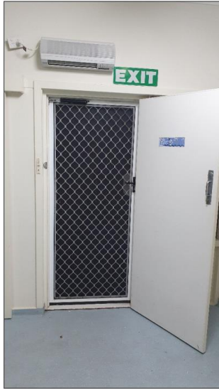
Ref # - 05 | Non-compliant EXIT door
