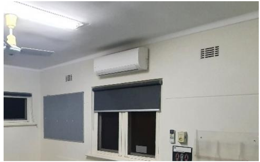
Ref # - 12 | Split Systems to be tested
