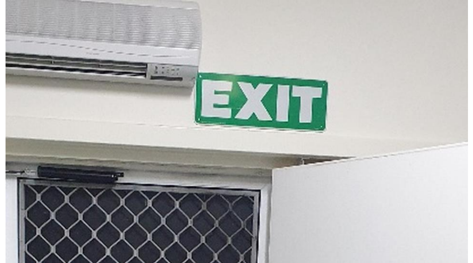
Ref # - 06 | Non-complaint EXIT signage
