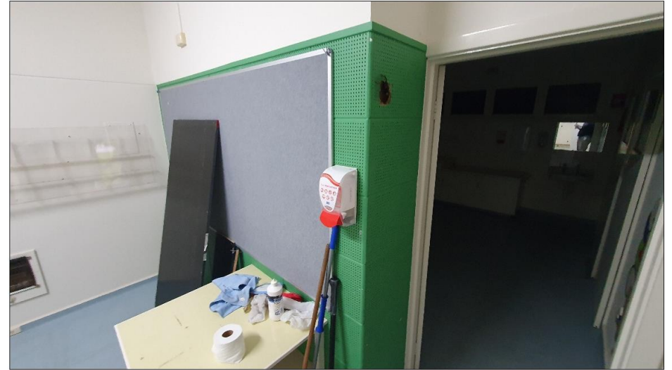
Ref # - 18 | Damaged acoustic panelling
