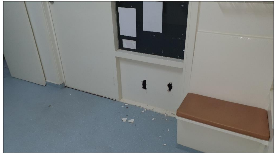
Ref # - 26 | Damaged panel at entrance
