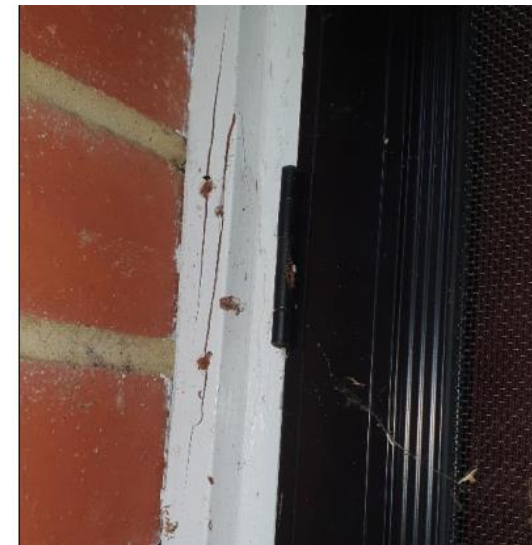
Ref # - 24 | Damaged Window and door frames throughout
