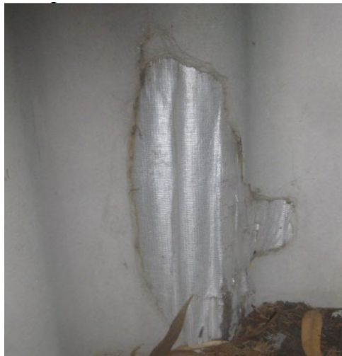
Taped fence hole from reverse side
