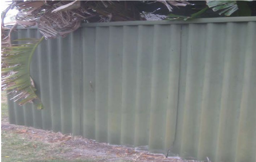
Painted ACM fence (with fasteners removed and with metal capping). Branches need trimming
